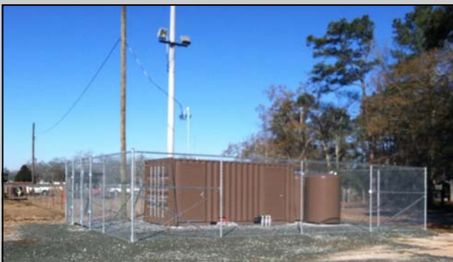
AS/SVE Equipment Compound
