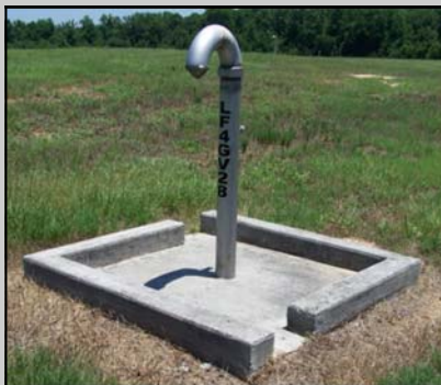
LF004 Passive Gas Vent
