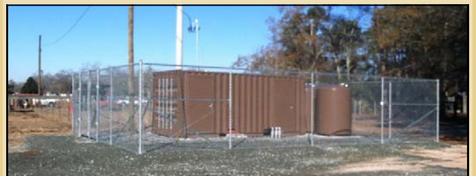
AS/SVE remediation equipment compound
