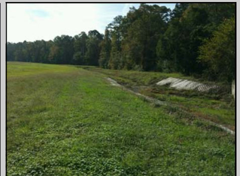
Stormwater Management Control (Run-On Diversion Channel)
