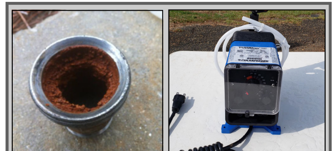
Iron deposition on extraction well caps at LF003 (left) and dosing pump for the iron deposition system (right).
