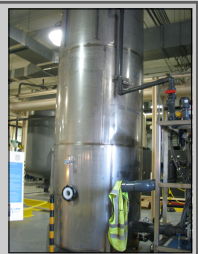
Close-up of Contact Tank.
