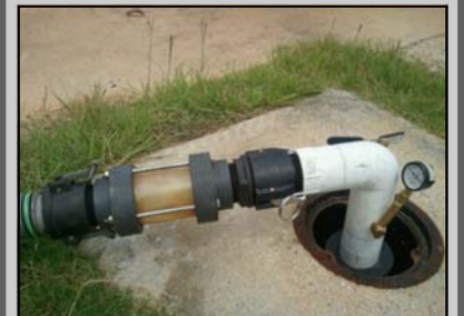
Close-up of Wellhead with EFR ® Connection
