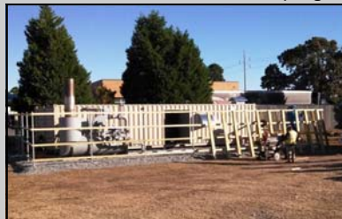
Treatment System for Extracted Soil Vapor
