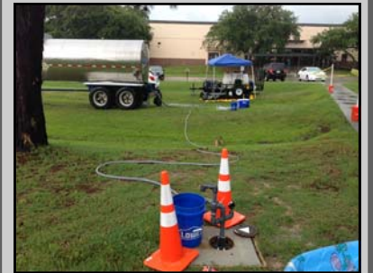
Typical Injection Well Header
