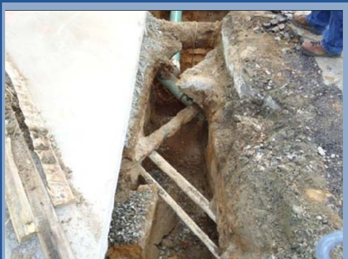
The numerous utilities present in the vicinity of the GBIA restoration sites present challenges to constructing, operating, and maintaining remediation systems.
