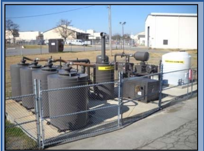
Vapor treatment system at SWMU 20.
